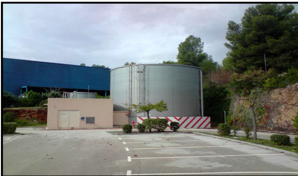
Autonomous tank with fire-fighting network.
